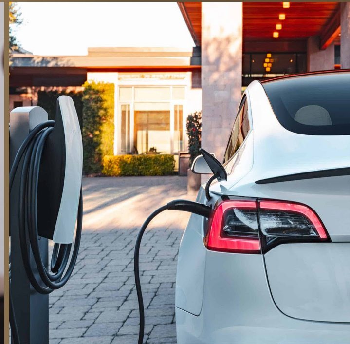
EV CHARGING SYSTEM
