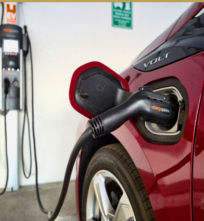
EV CHARGING SYSTEM
